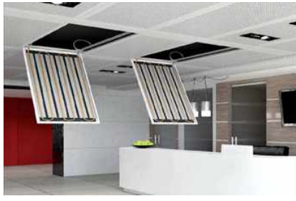
Radiant ceilings panels
