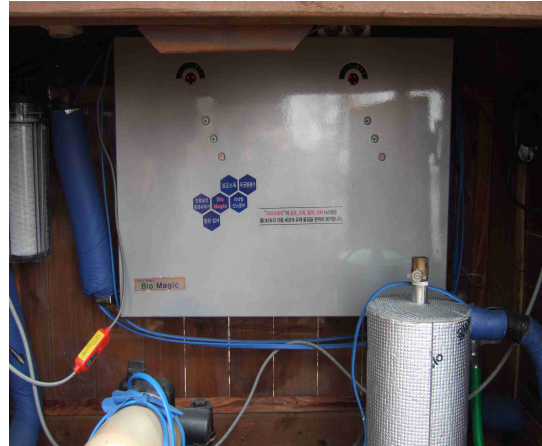
Fig. 2. Picture of ozonation system.
