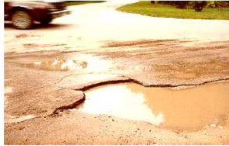
Condition 4: Safety Hazard
