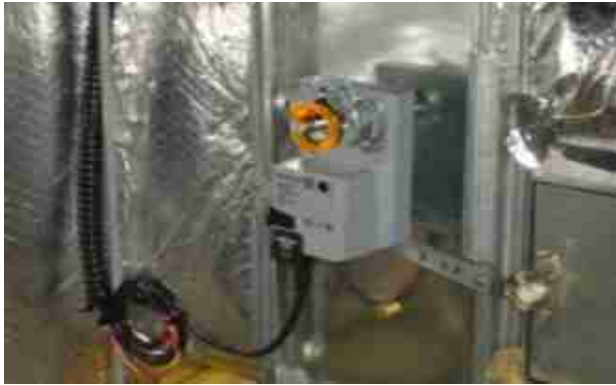
ZONE DAMPER 설치후
